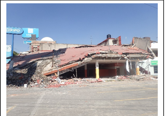
Photo.1 Example of collapsed building
